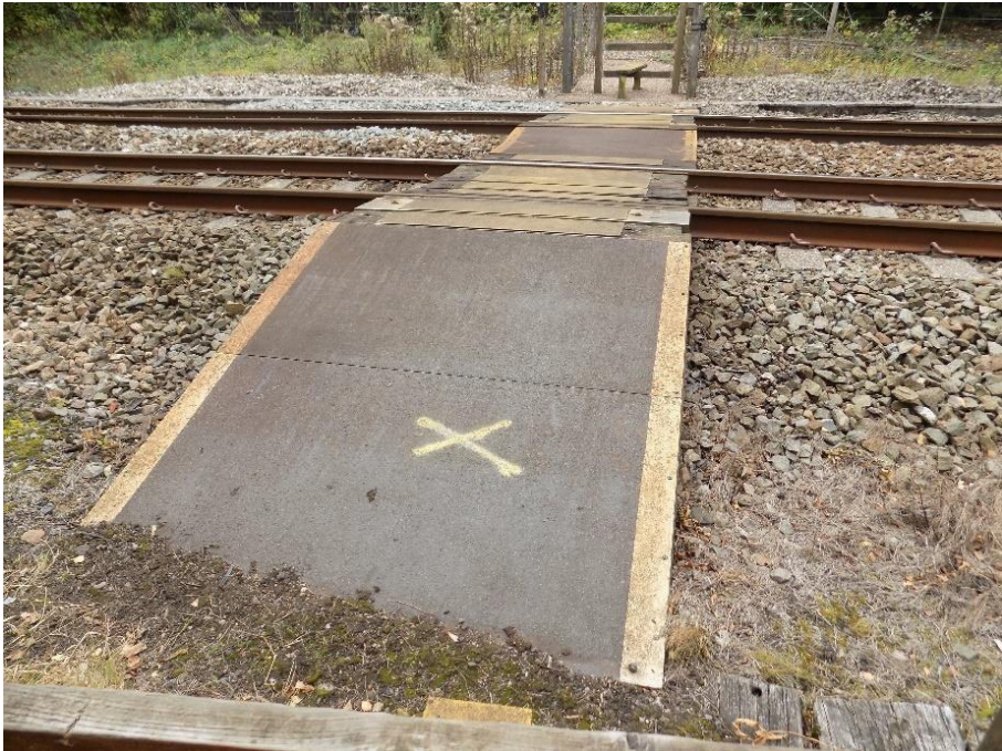
Figure 2-4.7: Level crossing deck
