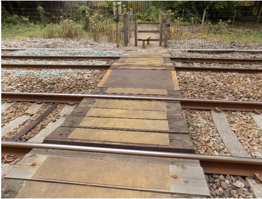
Figure 2-4.8: Level crossing deck
